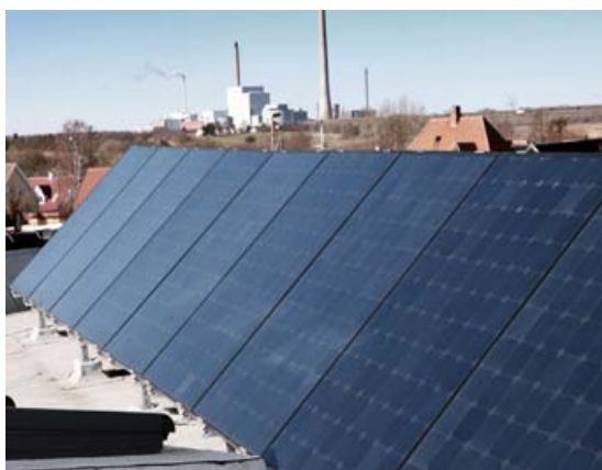
Solar panels on branch roof in Seden
